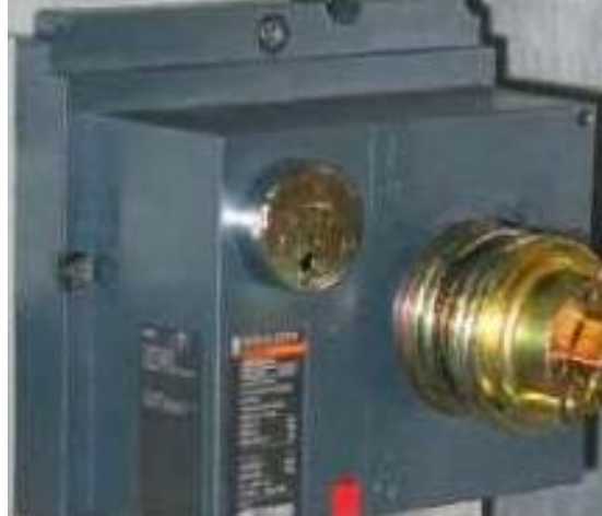
Figure 2-2: Lockout Key Location on Main Breaker (MTD0525)
