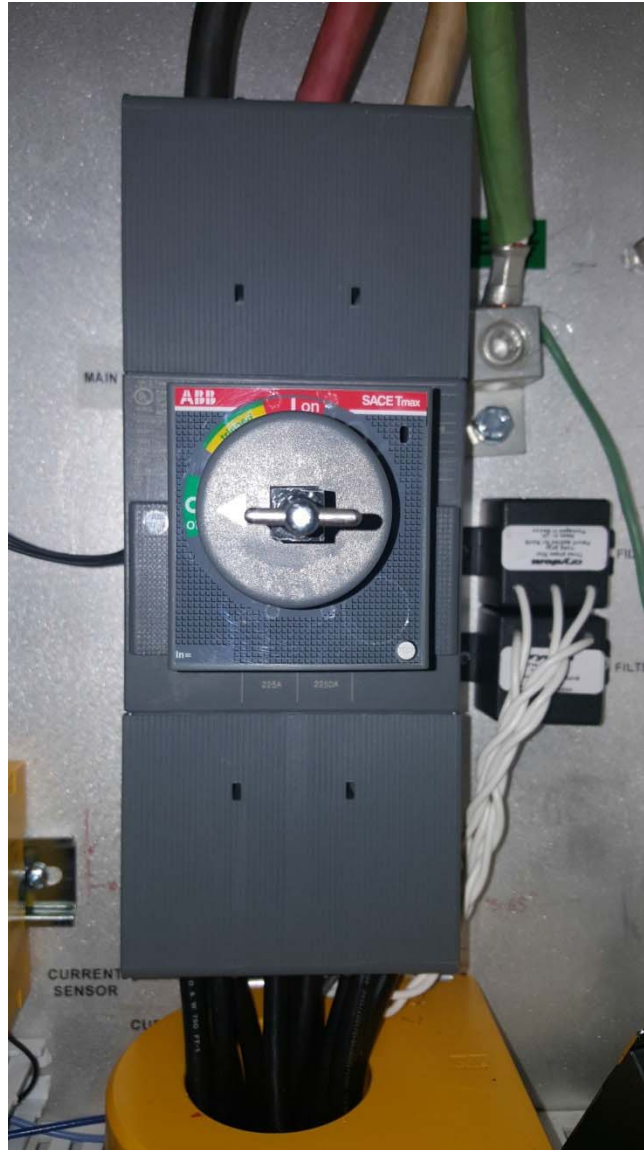
Figure 3-1: Main Circuit Breaker
