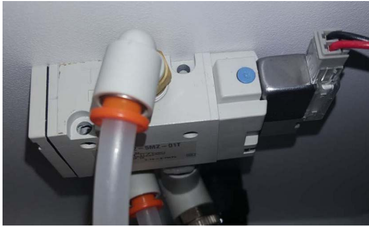
Figure 7-2: Isolation Valve Control Solenoid
